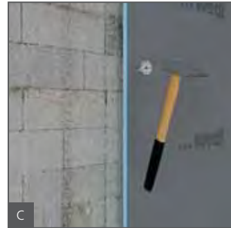
C Place wedi Tools metal dowels in the holes and hammer in after the mortar has fully dried.
